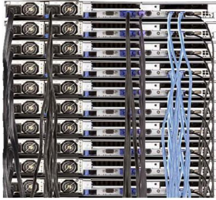
Ten 1U dual processor servers and the associated cabling.
